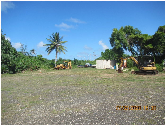
Photograph 6: IMG_1347: This photograph was taken facing southeast. Mr. Alo stated that the graded area in this picture is the extent of the fill placed on his property. Mr. Alo stated that the heavy equipment on the left side of the frame and vehicles in the background are out of service.
